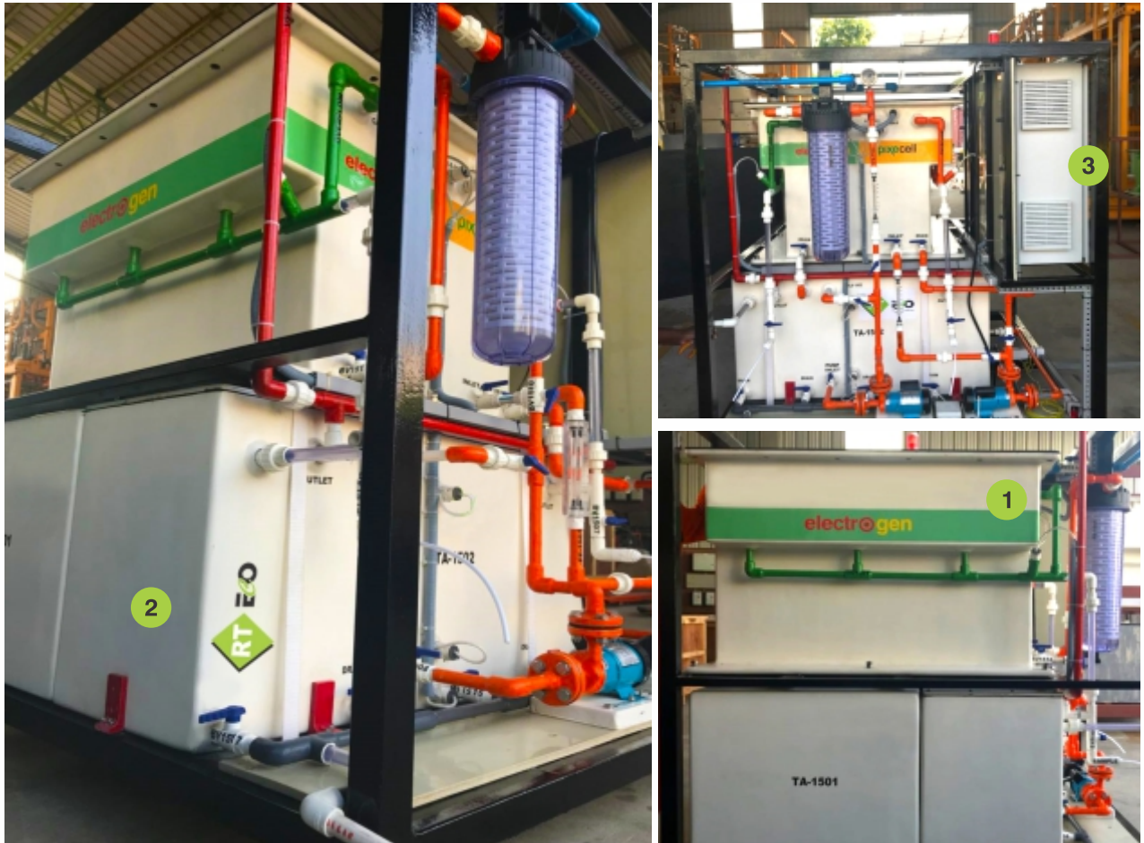
1 Electrolyzers - for Electro-coagulation and electro-oxidation
