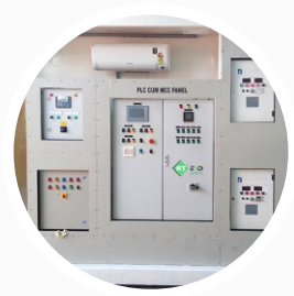
MCC & PLC Panel
