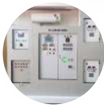
MCC & PLC Panel
